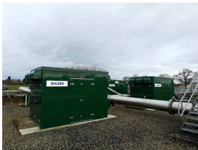
The Rushmoor facility serves more than 50'000 - four HST20-6000-1-125-40 turbocompressors were installed as replacements for ageing inefficient and unreliable blowers.
