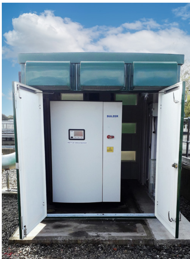
HST turbocompressors installed in bespoke GRP enclosures which offers flexibility and savings on civil works costs.
