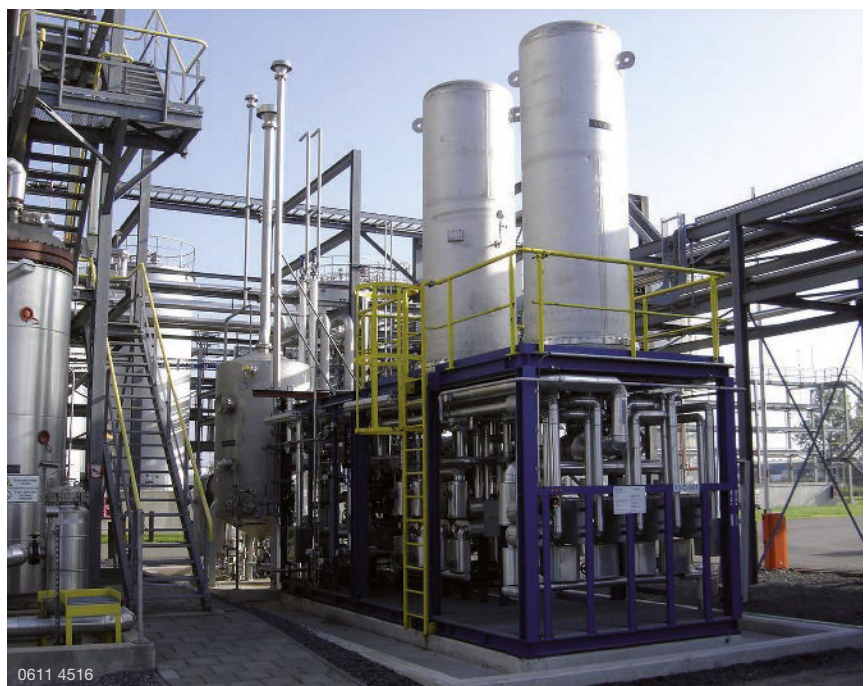
Skid mounted PERVAP™ membrane plant
